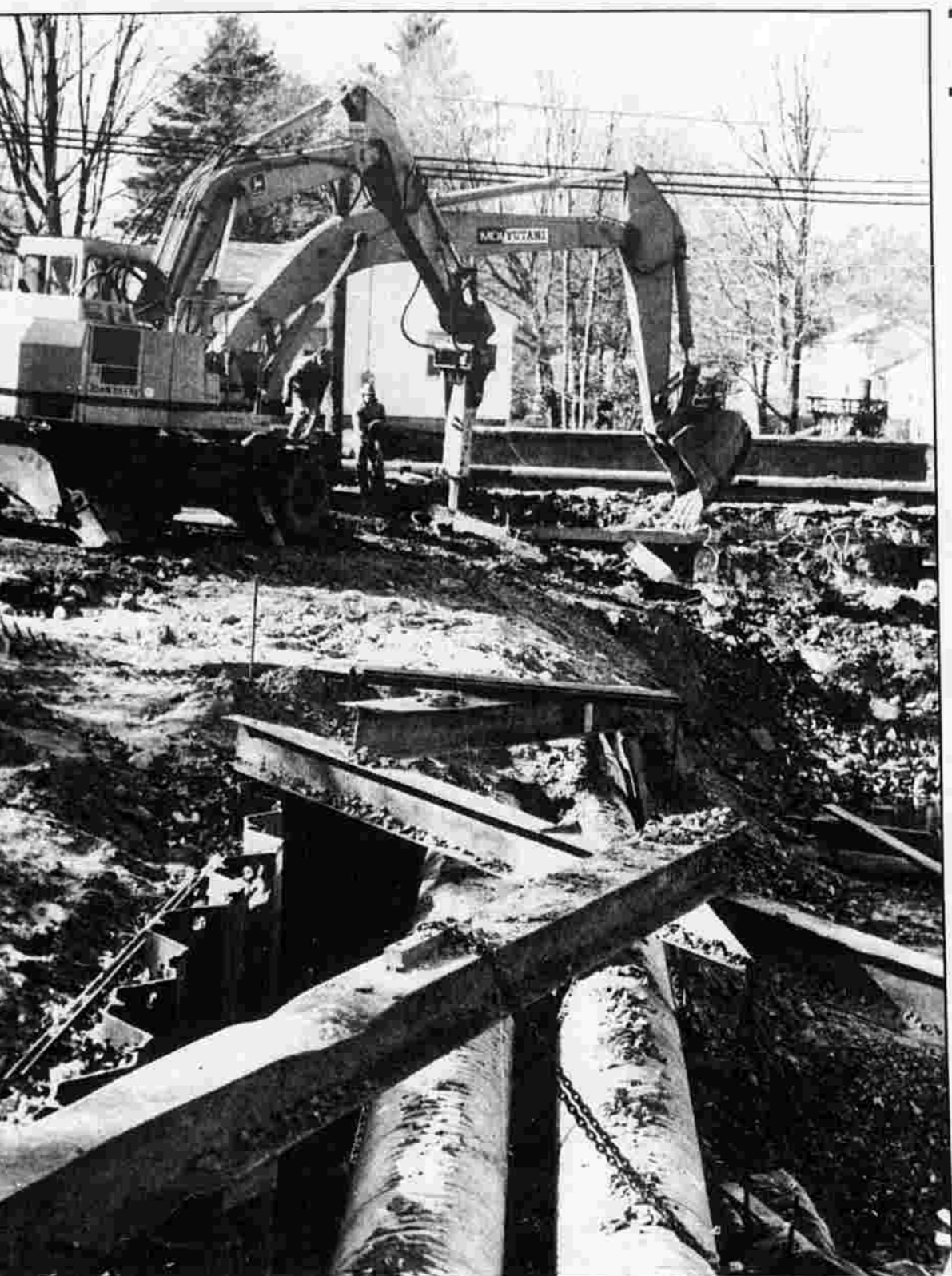
Heavy duty construction — Workers for Central Paving of South Windsor prepare to install water mains at the intersections of Autumn, Charter Oak, Highland and Oak Grove Streets.
